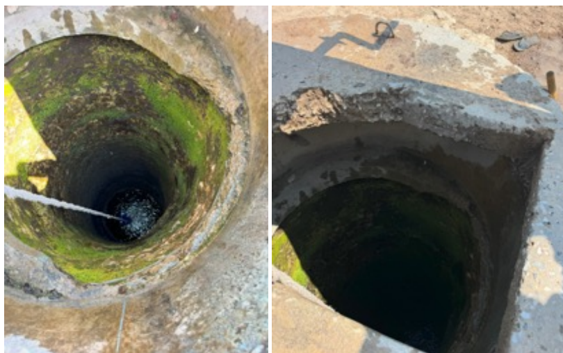
Figure 5-4: Safety risk – uncovered community well
